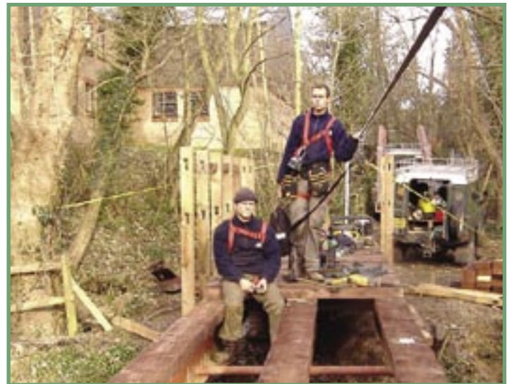
Anthony Hart and Dave Tonge putting wooden cladding onto the steel frame at Forest Row
